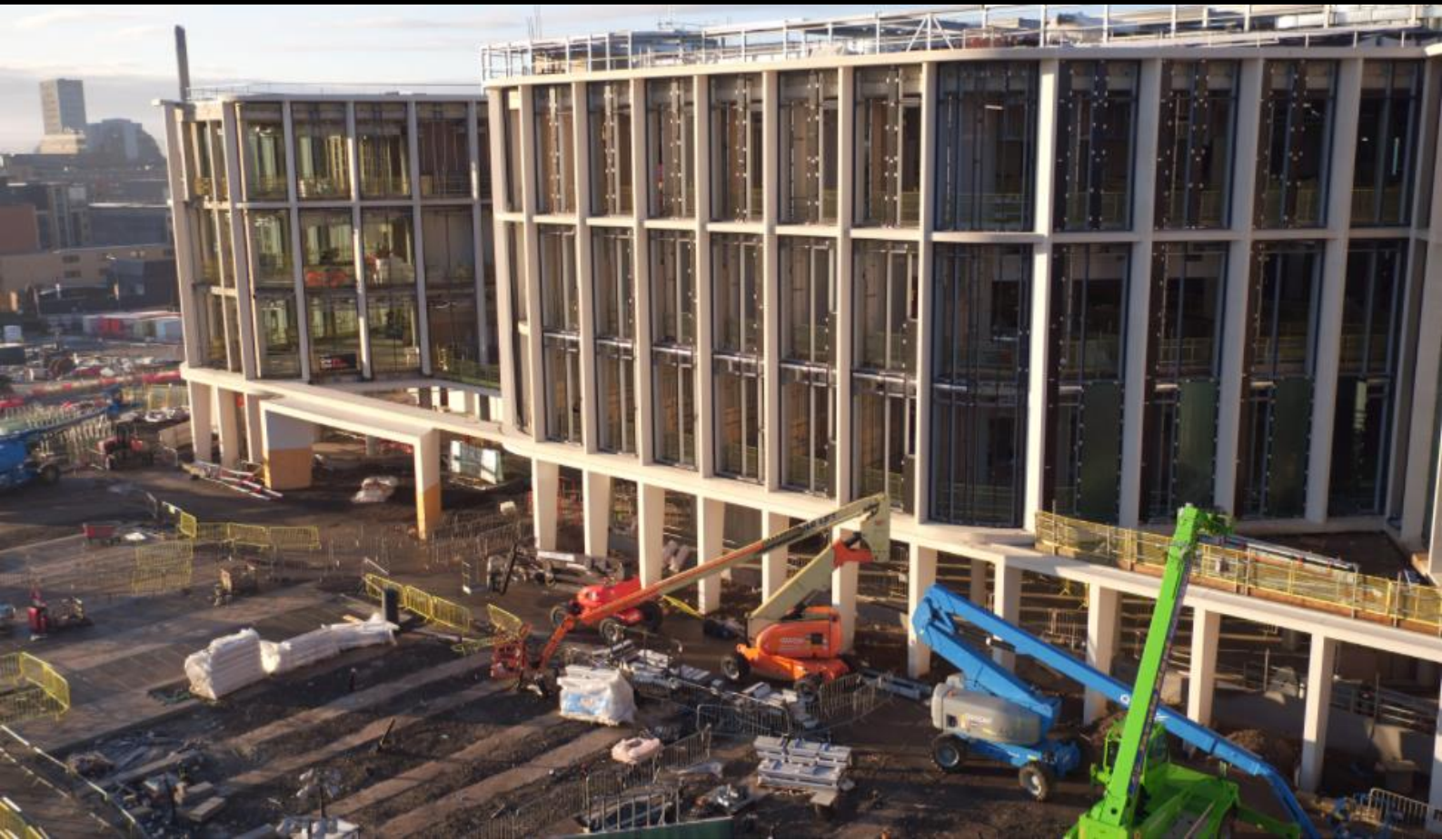
The East elevation of the Research Hub including landscaping works for University Square
